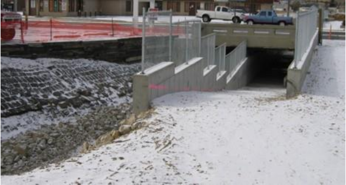
Figure 9. Pedestrian tunnel passing underneath Harrison Avenue, linking the MSD trail between east and west Butte.
