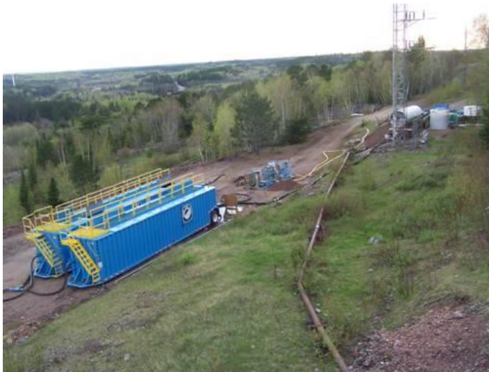
Figure 2. Overview of treatment system
