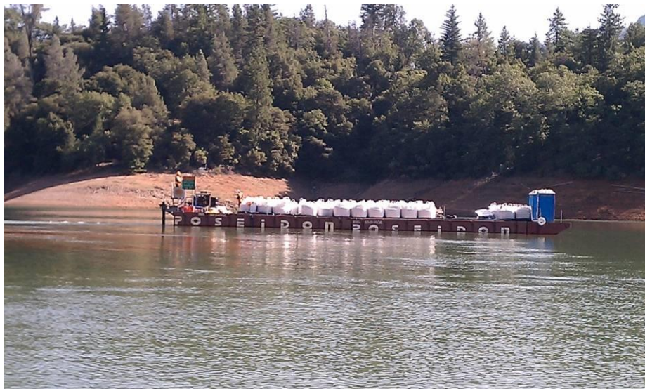
Figure 5. Barge delivery of supersacks filled with organic substrate or other construction materials (e.g., drainage gravel and rip rap)
